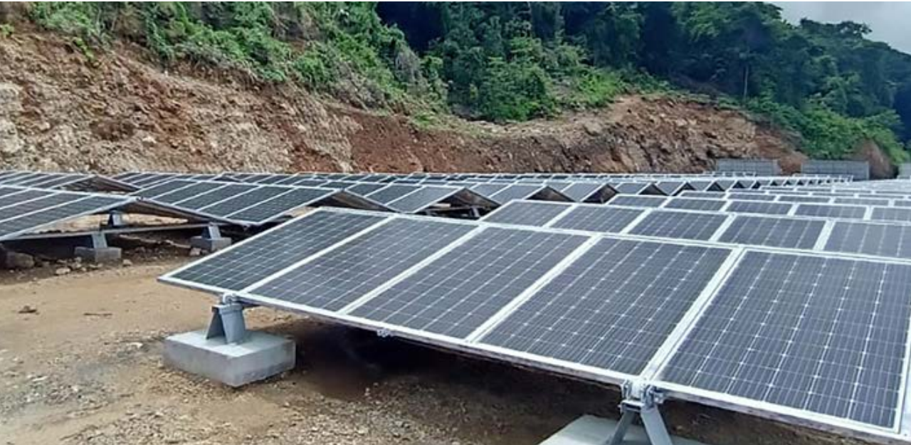
▲ Solar panel at Wetar Copper Mine
